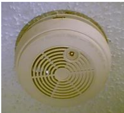
Residential ceiling-mounted smoke detector
